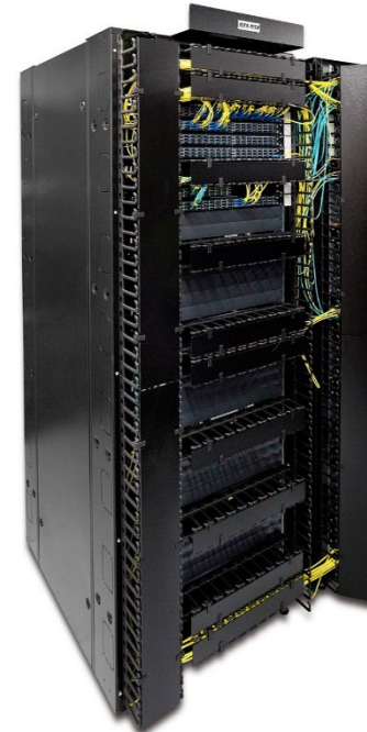
patch location rack
