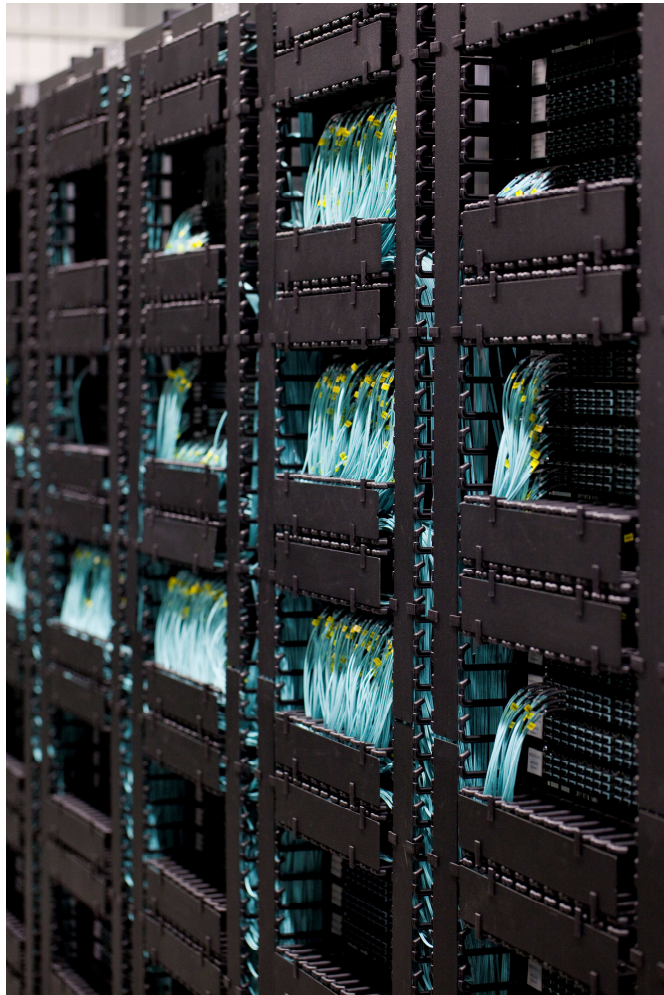
Best Practise DC High-Density Patch Location built of former OSI „Data-Center-Rack“
